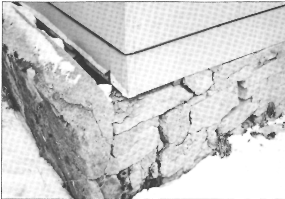
Commentary Figure 304.5 MAJOR DAMAGE TO A FOUNDATION WALL This foundation is crumbling. Failure to repair it will eventually lead to its collapse.
